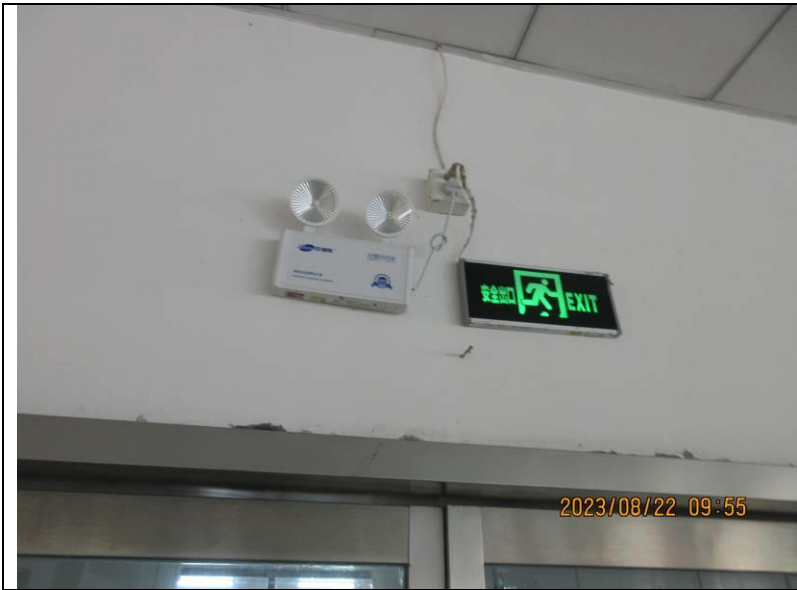
Exit sign and Emergency light
